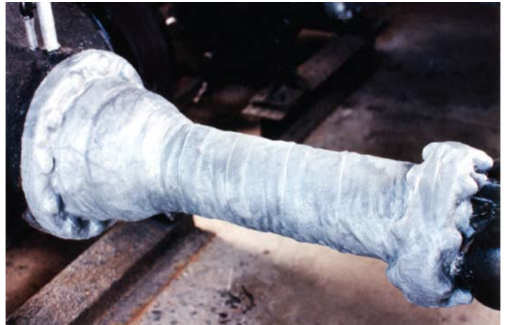
A sweating meter run pipe protected with #2A Wax-Tape demonstrates the tape's ability to protect in wet conditions.
