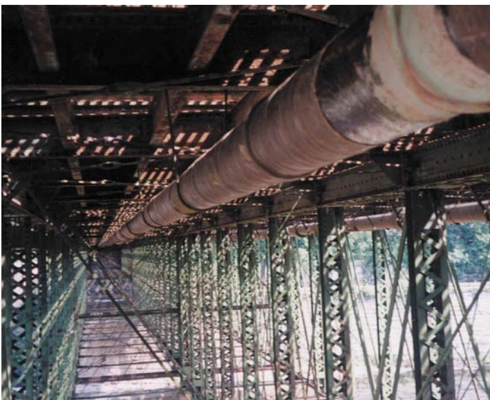
Sometimes sandblasting is awkward and environmentally questionable, particularly when the work is directly over a river or stream. Wax-Tapes do not require sandblasting.
