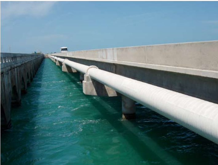
White Wax-Tape Primer and #2W Wax-Tape (white) were used over this water location, because sandblasting the pipe would have raised environmental concerns.
