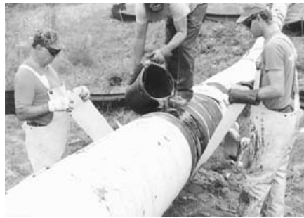
Innercoat wax coating being applied directly to the pipe surface using the Guard-Wrap wrapper as a "granny rag."
