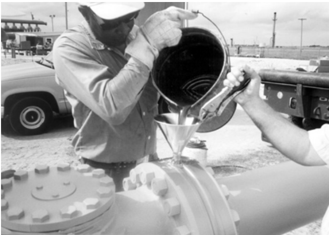
Flange filling is the process of pouring hot Innercoat between the flange faces to prevent corrosion.
